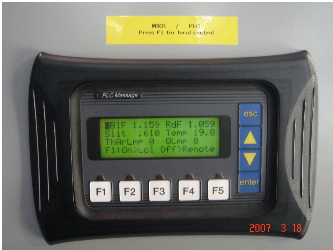
Figure 11. Local control panel (showing remote mode screen).
